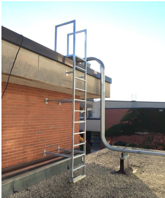
Picture 7 – Roof ladder. Not anchored to the roof.
