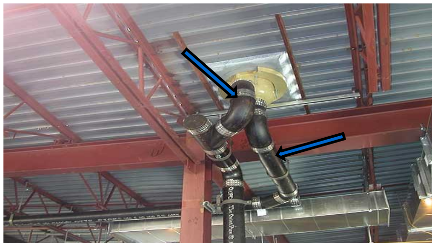
Picture 16 – Main roof drain and overflow drain have independent drainage system and discharge below roof
