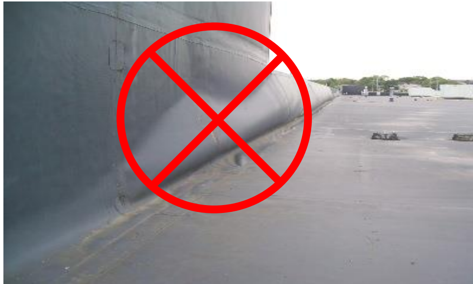
Picture 14 – Roof membrane used as wall finish is not acceptable by this guideline.
