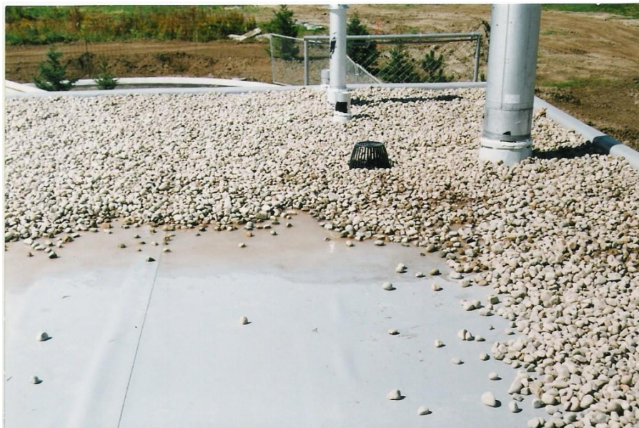
Picture 10 – Ballasted roof with washed or blown ballast exposing roofing membrane
