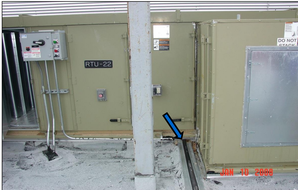
Picture 9 – This roof expansion joint will not function as intended
