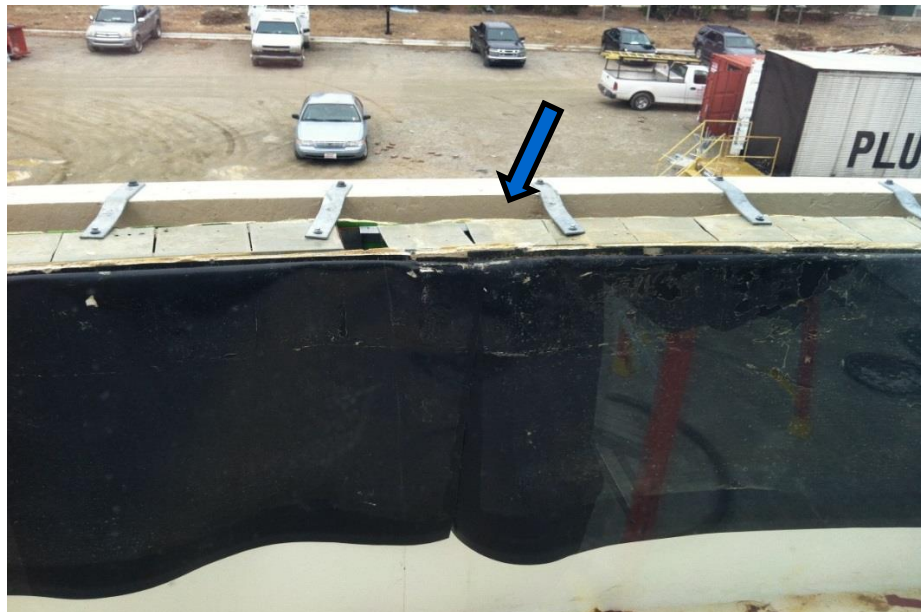
Picture 11 – The wall cavity must be protected from water intrusion.
