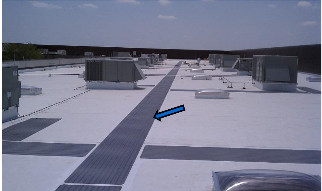
Picture 6 – Rooftop walk-pads and at equipment service panel.
