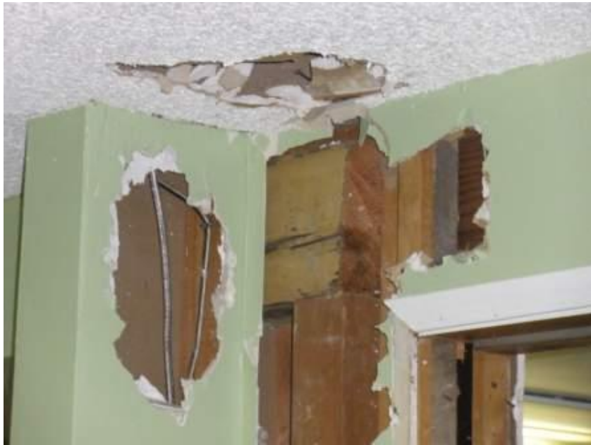
damaged and friable popcorn ceiling material
