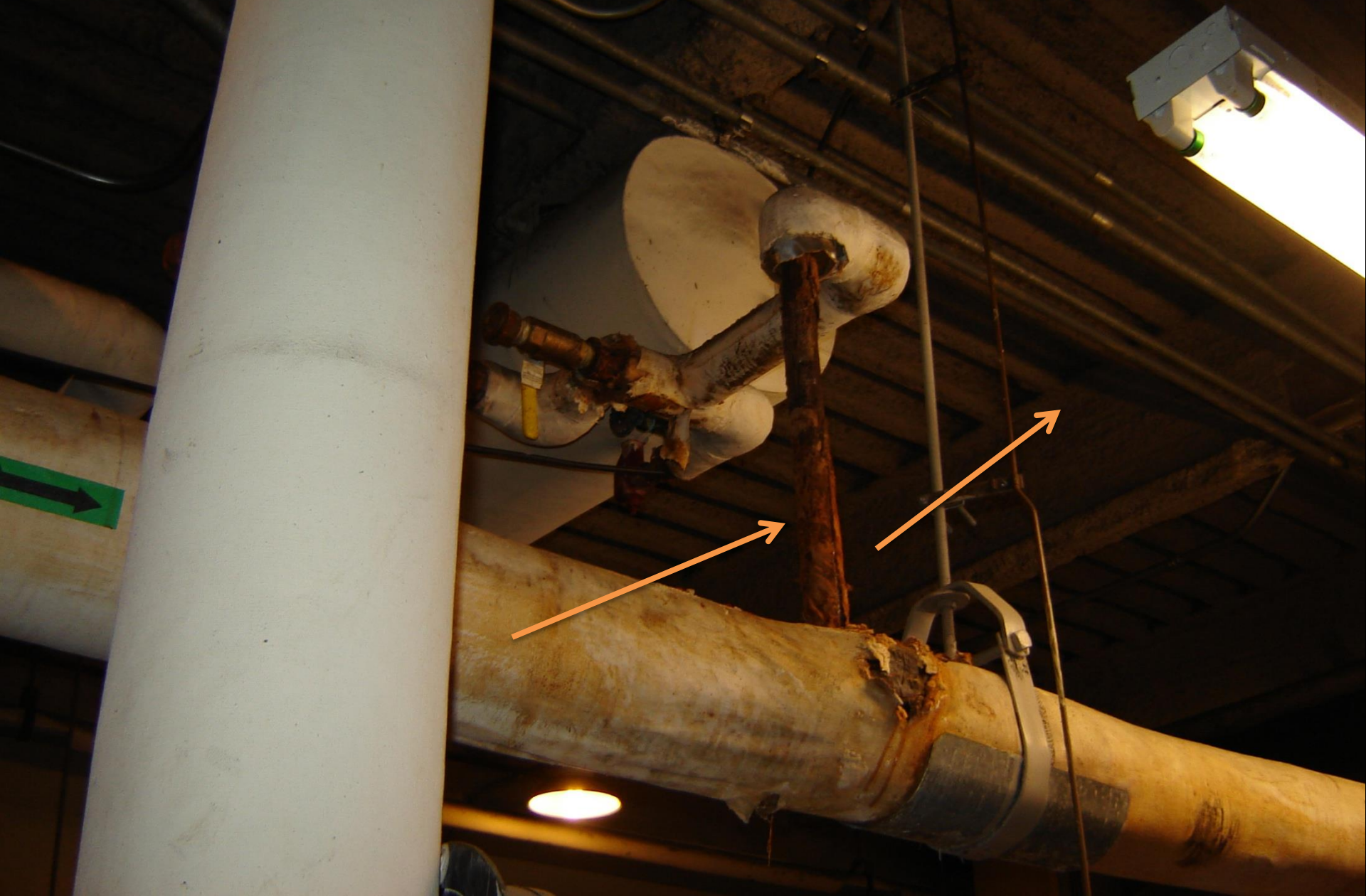
DOA – Administration – Sprayed on asbestos fireproofing releasing from structure and HVAC piping in poor condition.
