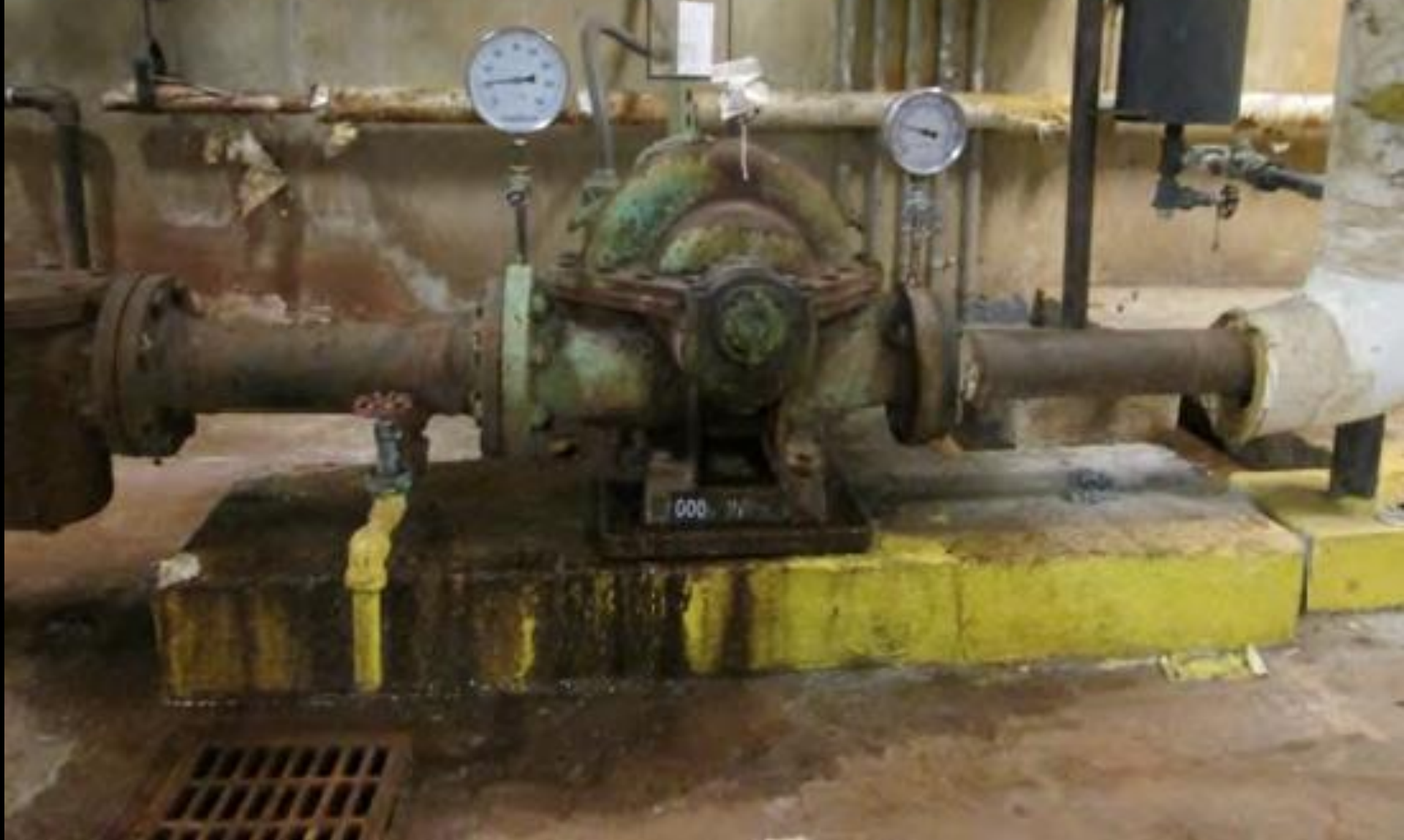
UNCC – Atkins – Hot water pumps and tank past life expectancy causing leaks and scaling .
