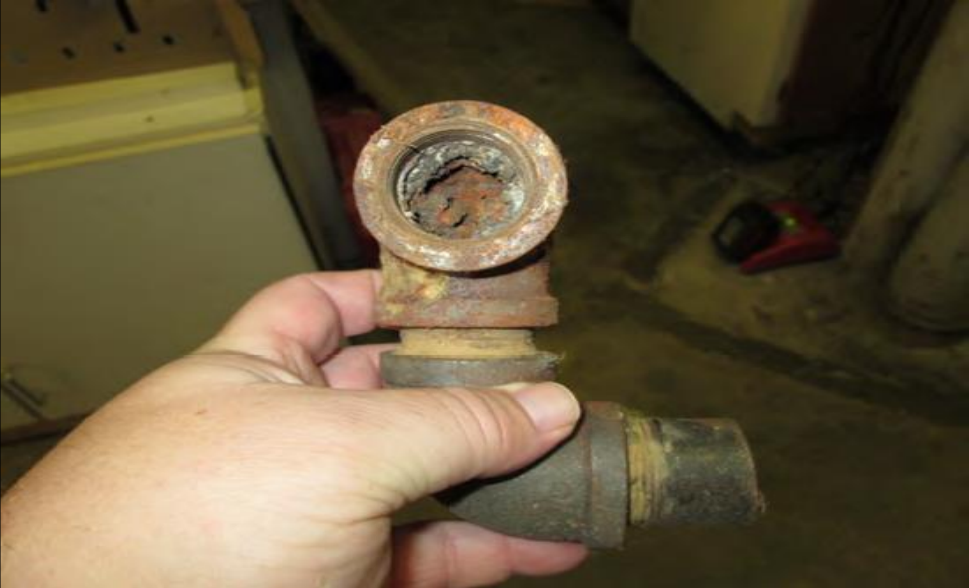
UNCC – Atkins - Hot water closed loop for heating showing signs of deterioration and massive scaling .
