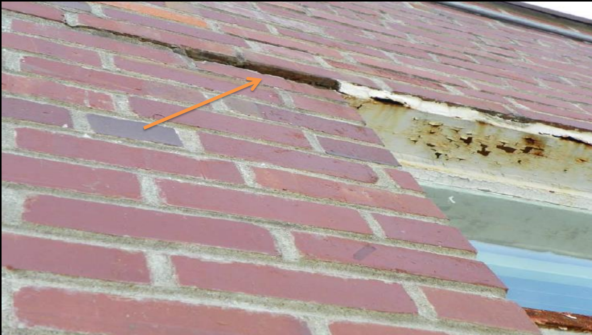
DPS – Dobbs Youth Development Center – Rusting lintels above windows causing structural problems. Typical across the state.
