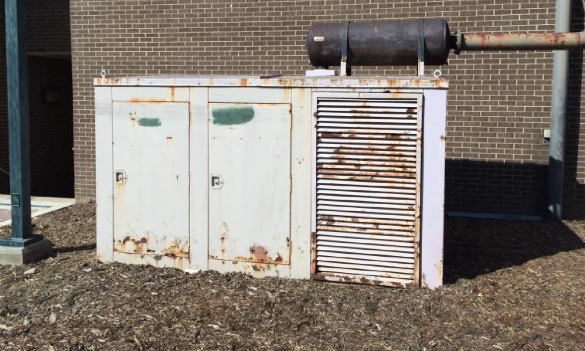
ASU – Health Services – Emergency generator out of service.
