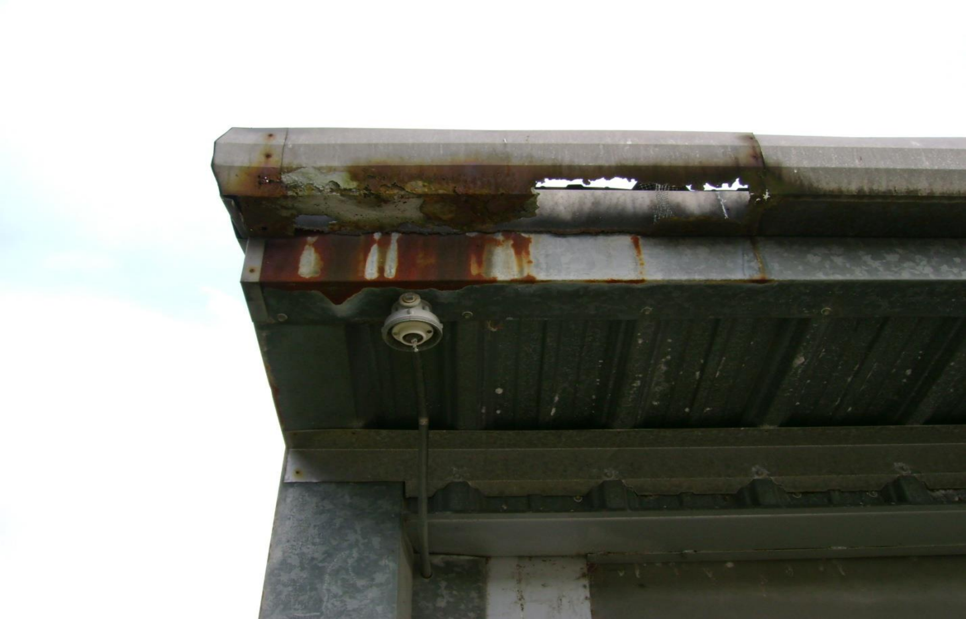
DHHS – Caswell Center – Gutter rusted through which causes roof water to pond against the building.
