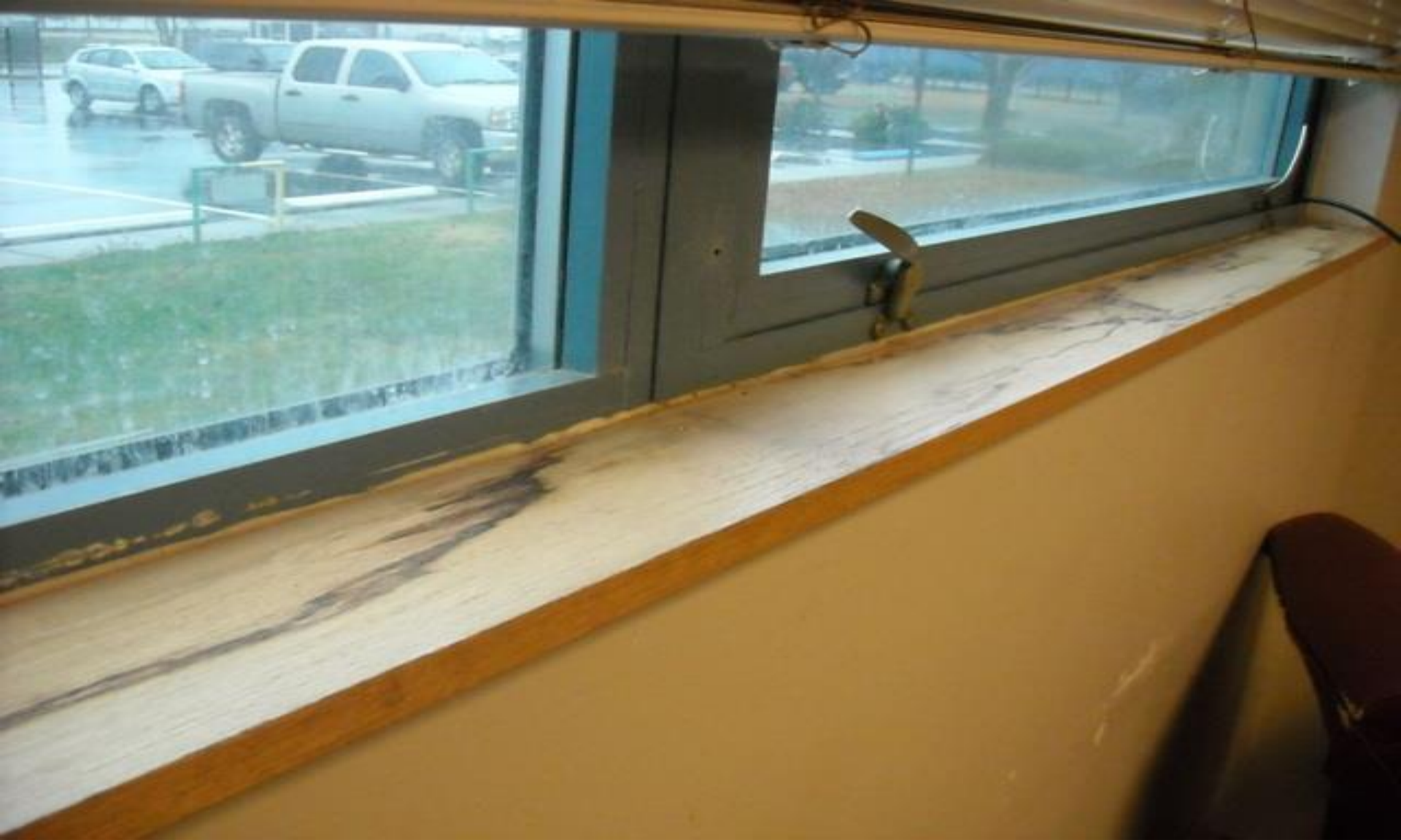
DPS – NCNG – Clinton Armory – Water infiltration through windows.
