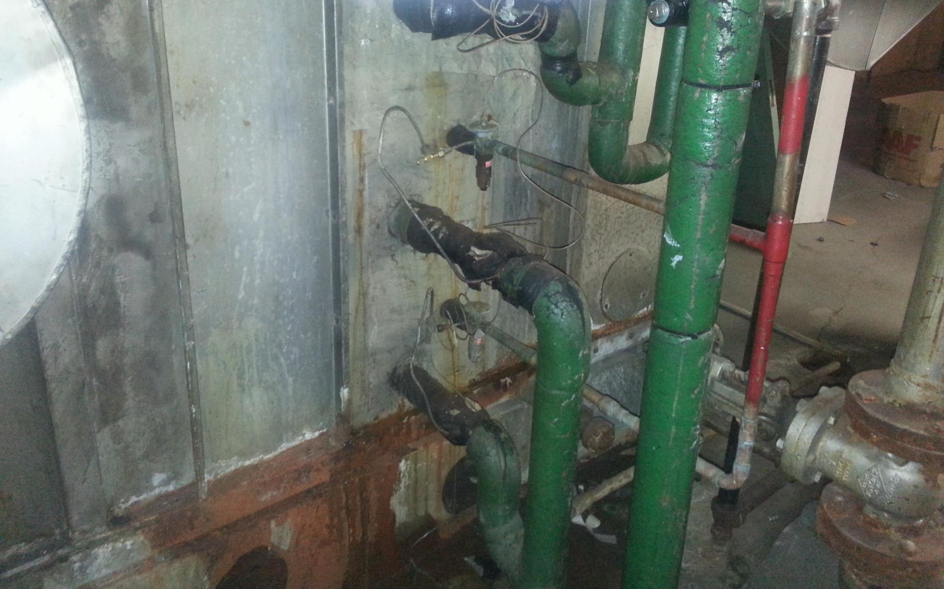
DOA – Shore – Corroded piping and equipment past useful life.
