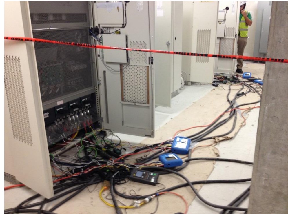
100 KW UPS under test
