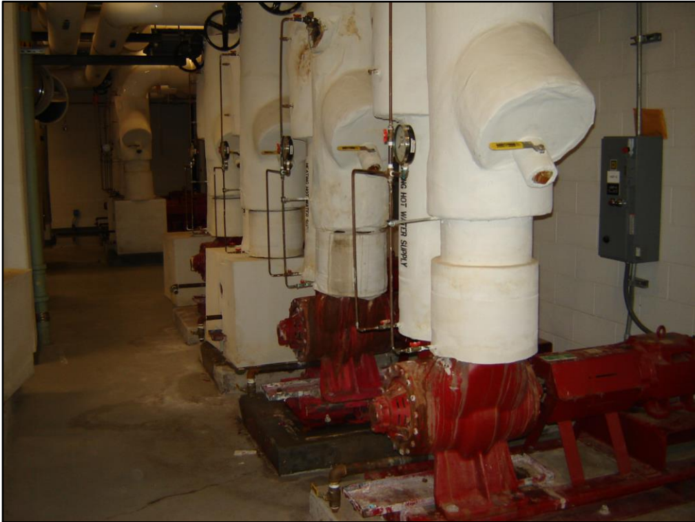
These are the pumps located on the other side of the open wall. (next)
