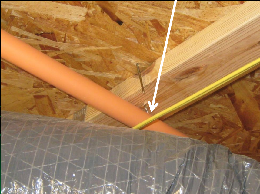
Nail in pipe
