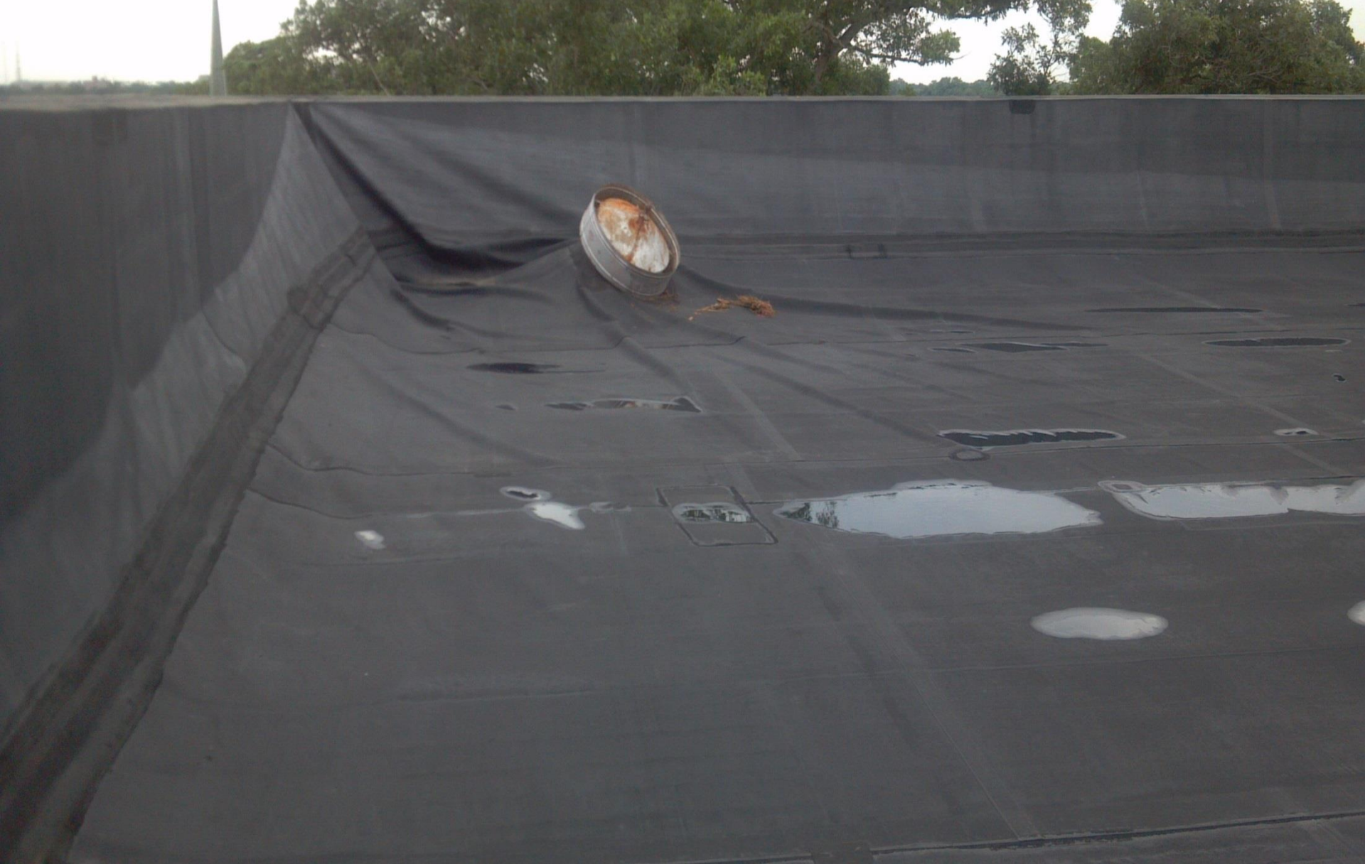
DHHS – Dix McBryde – EPDM roofing membrane failure.
