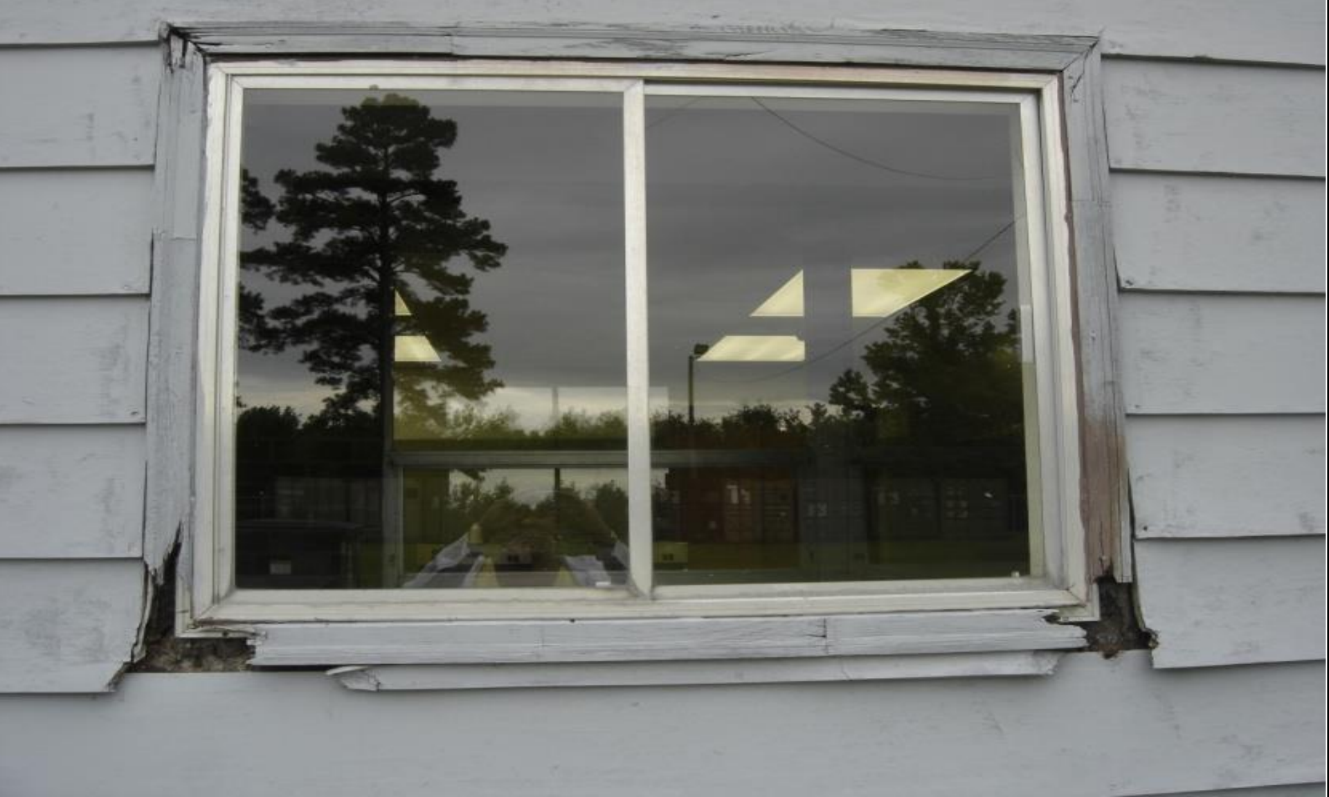
DPS – NCNG – Beulaville – Water infiltration due to rotting siding and window trim.
