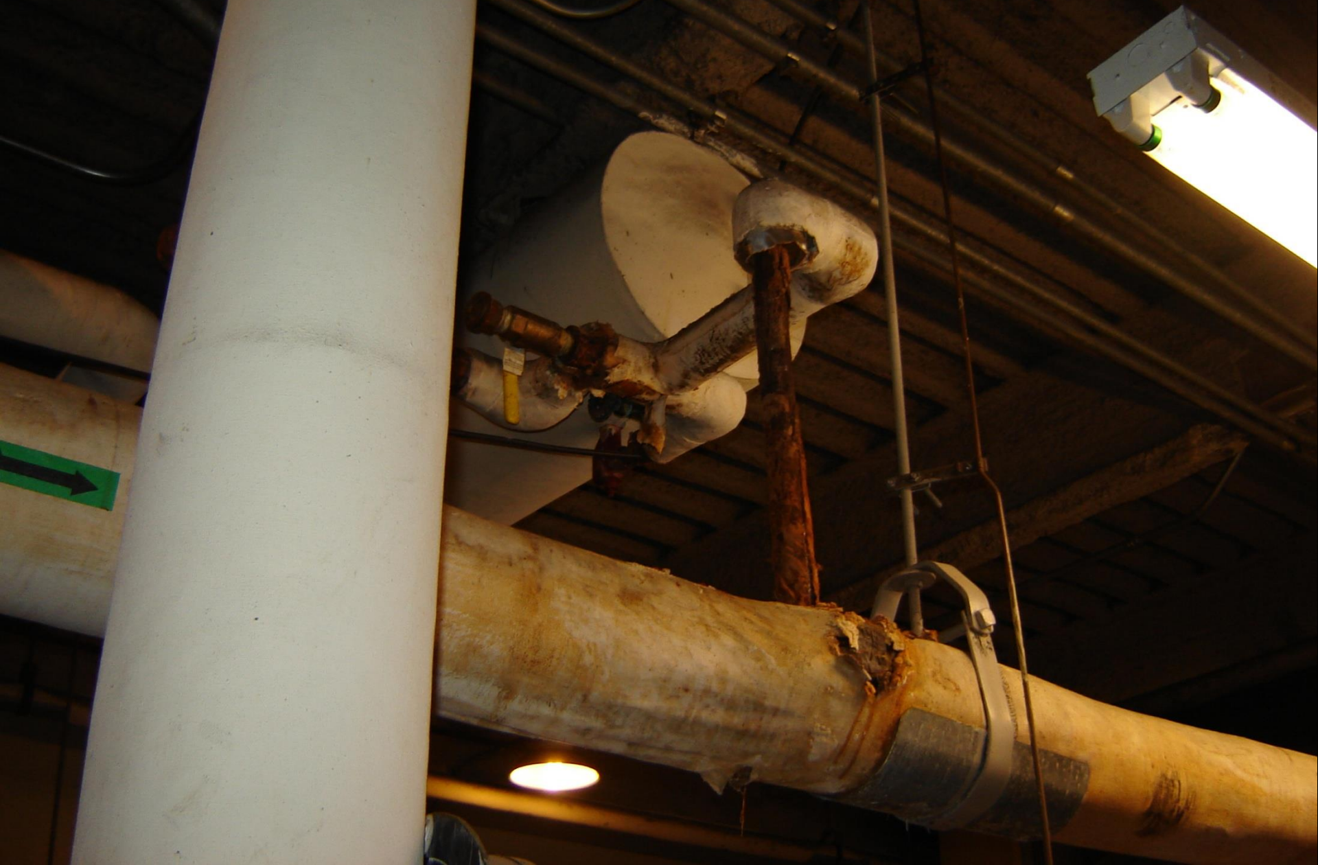
DOA – Administration – Sprayed on asbestos fireproofing releasing from structure and HVAC piping in poor condition.
