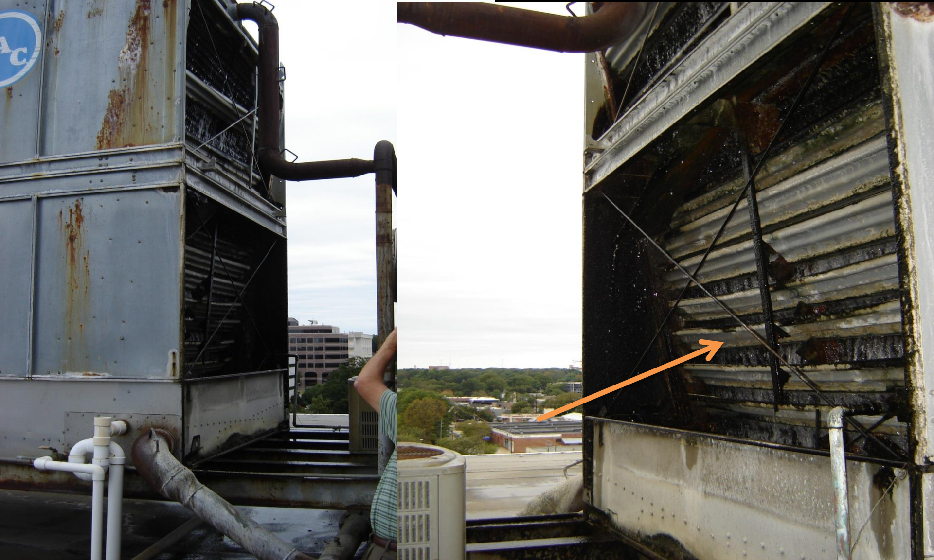
DOA – Shore Bldg – Cooling tower past is useful life. Rusted and broken supports.
