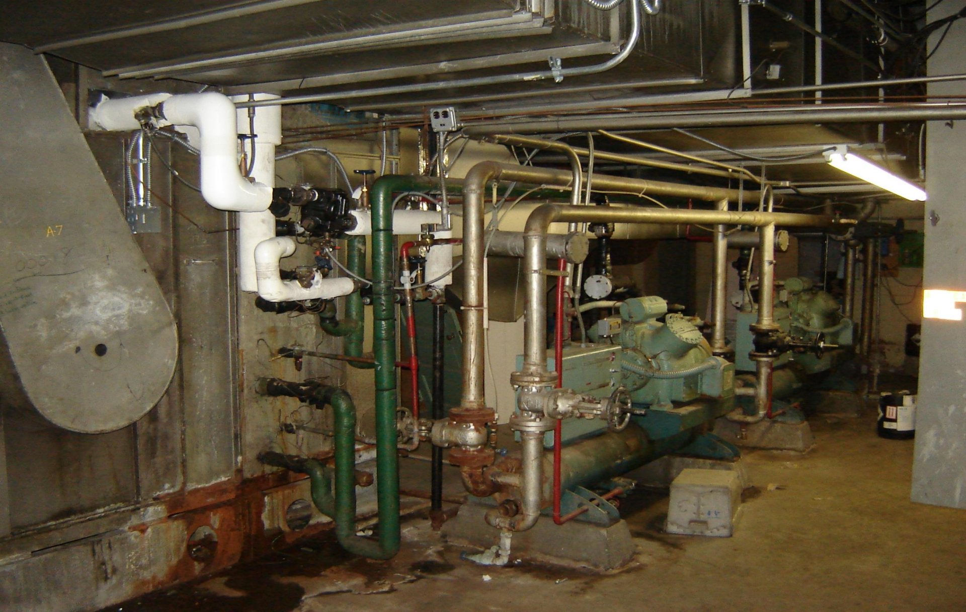
DOA – Cooper – HVAC equipment in poor condition. Installed in 1940's.
