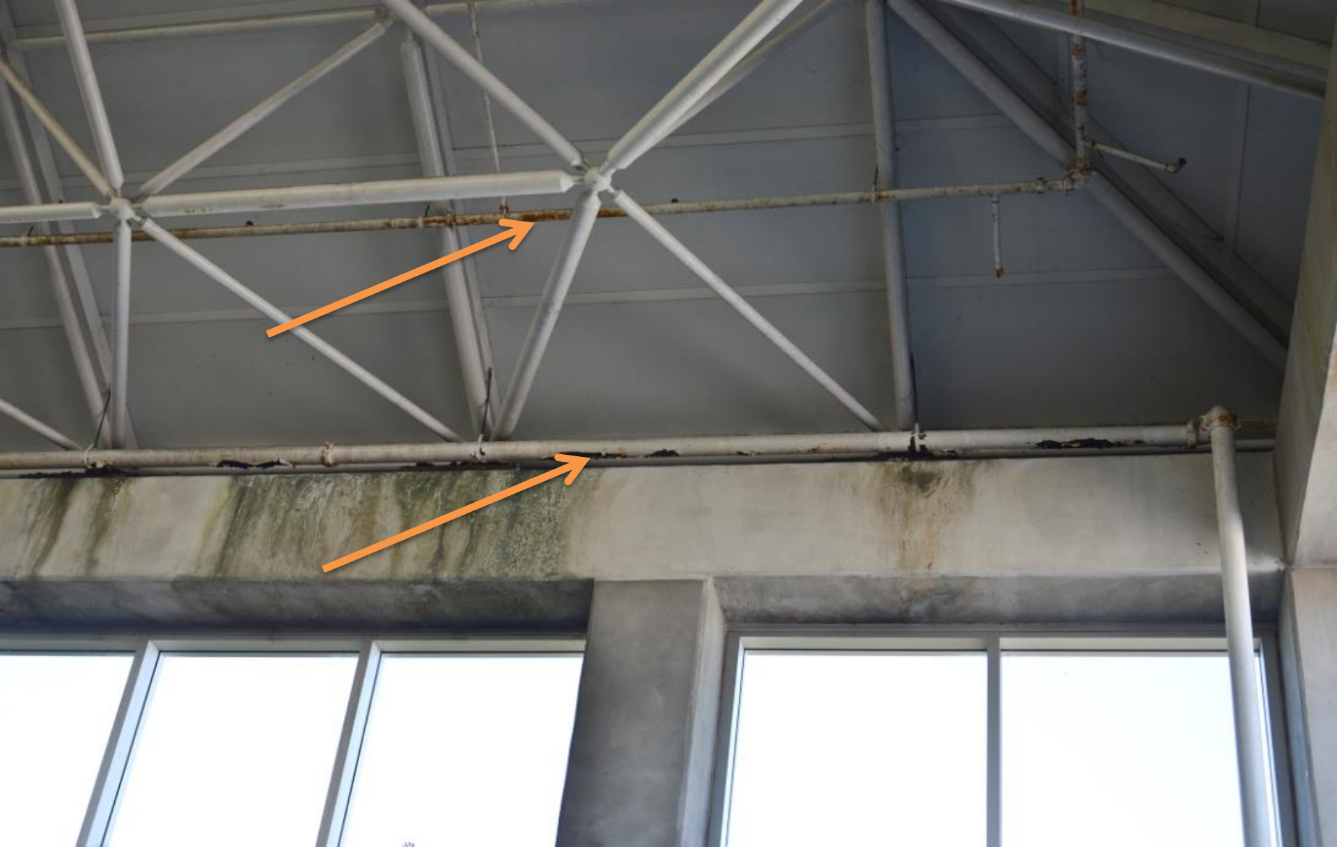
DENR - Fort Fisher Aquarium – Fire sprinkler pipes in the conservatory are corroding as a result of exposure to the salt air.
