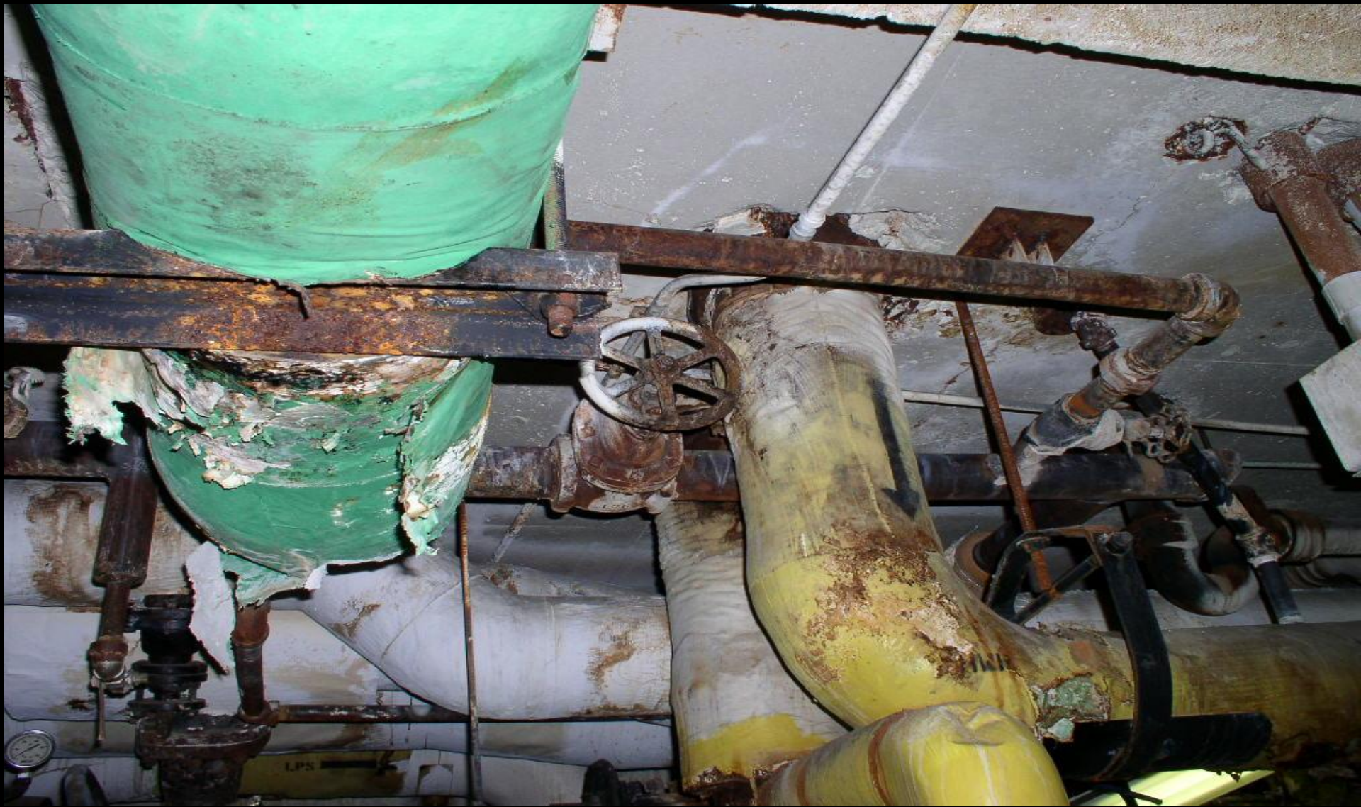
UNC-CH – MacNider Hall – HVAC system is deficient and poor shape.
