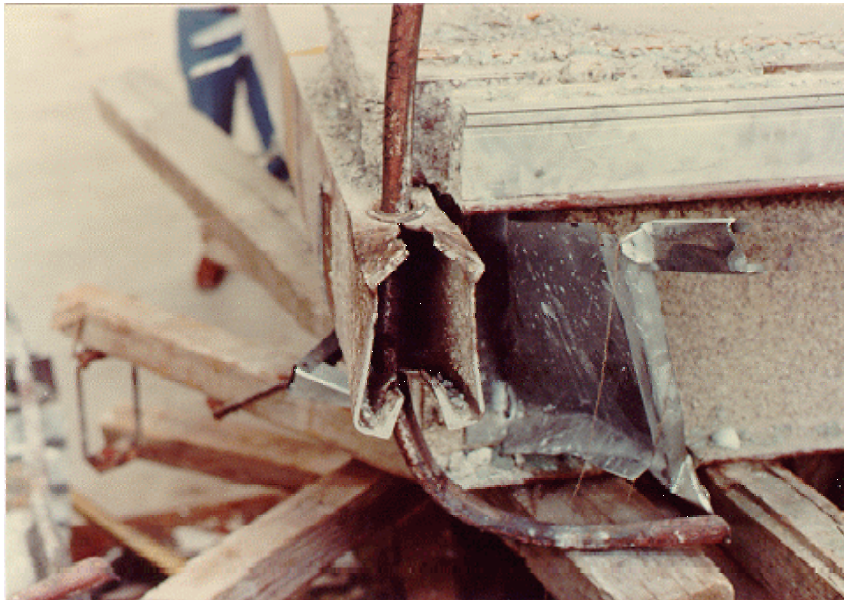
114 people killed Attachment detail of steel walkway June, 1981 Kansas City, Missouri
