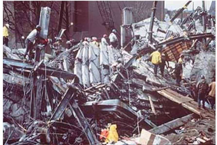
28 workers killed Lift slab construction April, 1987 Bridgeport, Connecticut
