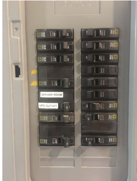
Photo 4: Elec. Panel Finance Office Hall
