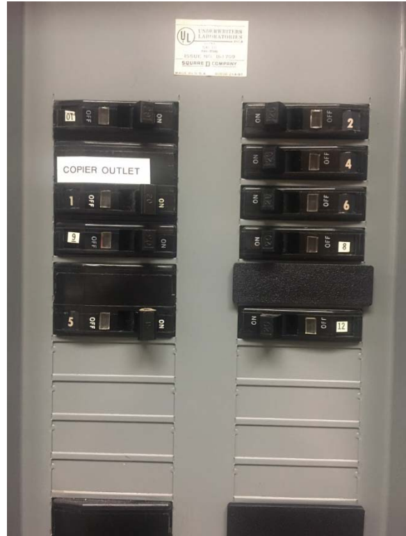
Photo 6: Electrical Panel Finance Office Room
