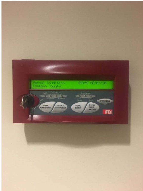
Photo 15: Sub Fire Alarm Panel (First Floor)
