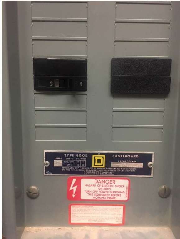
Photo 7: Electrical Panel Finance Office Room
