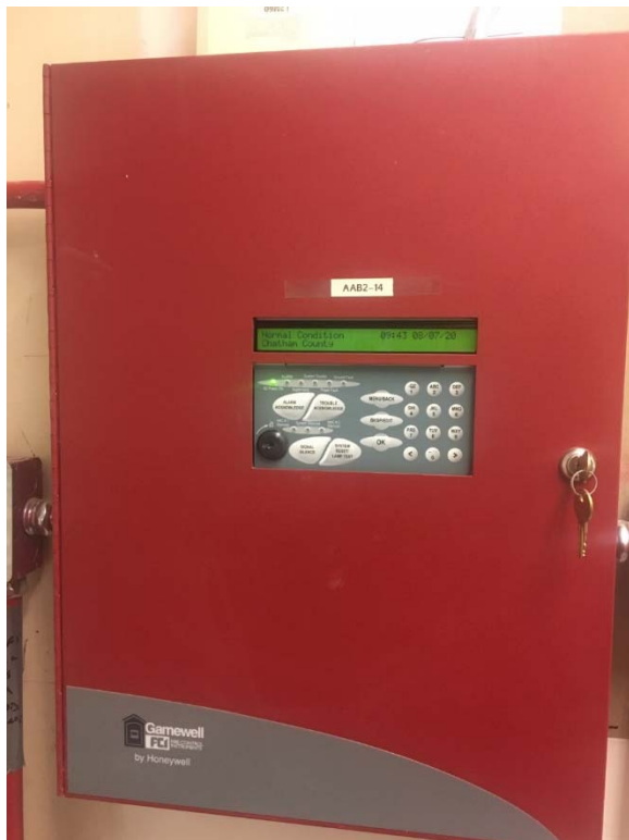
Photo 1: Fire Alarm Control Panel
