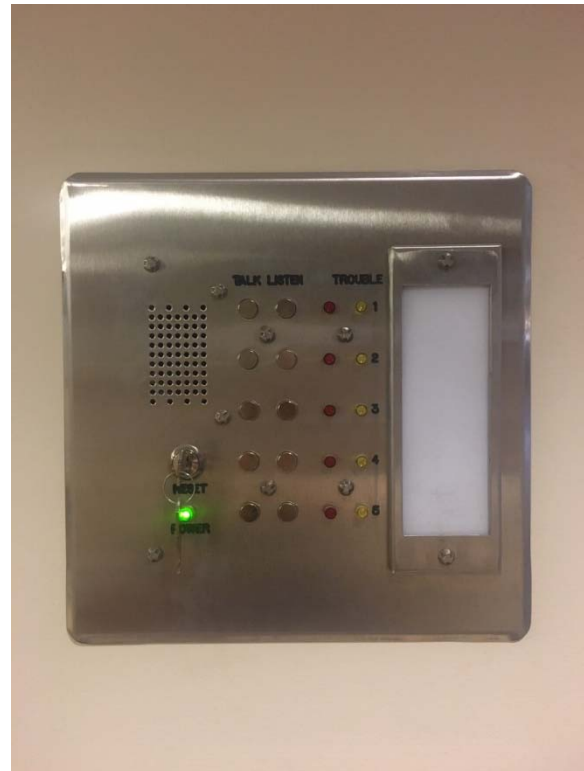
Photo 16: ARA Communication Panel (First Floor)
