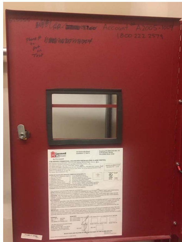
Photo 2: Fire Alarm Control Panel Door
